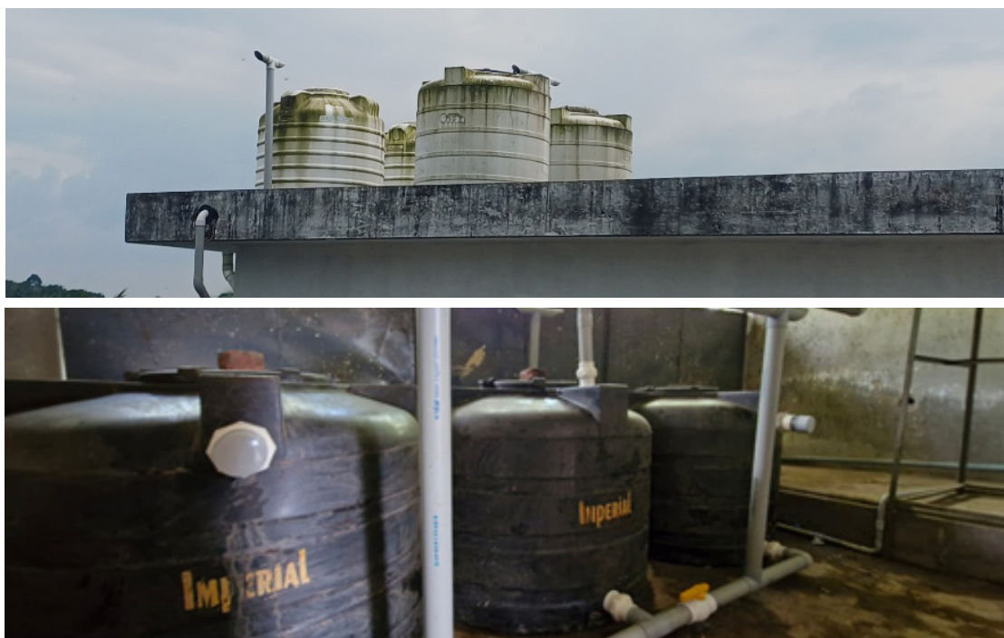
Fig 5.3 Water storage tanks
