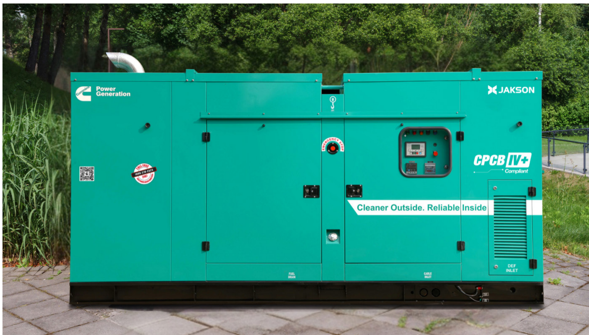
Fig 4.27 College Diesel Generator Unit
