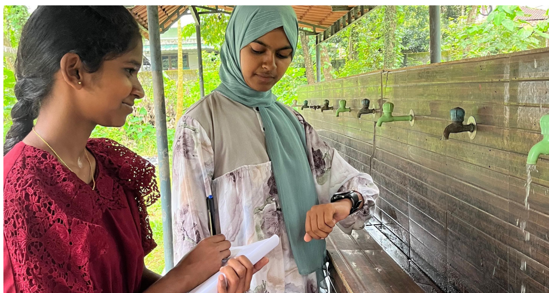
Fig 5.5 Water Supply Fixtures and Infrastructure- Hostel
