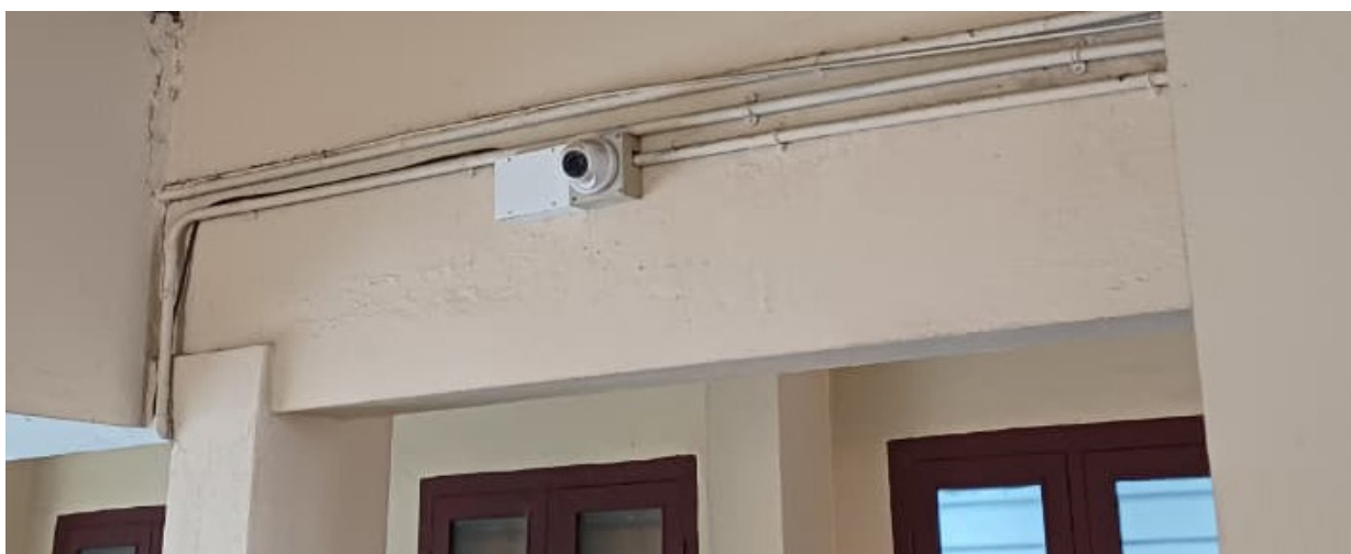
Fig 8.7 CCTV Surveillance System for College Event Monitoring
