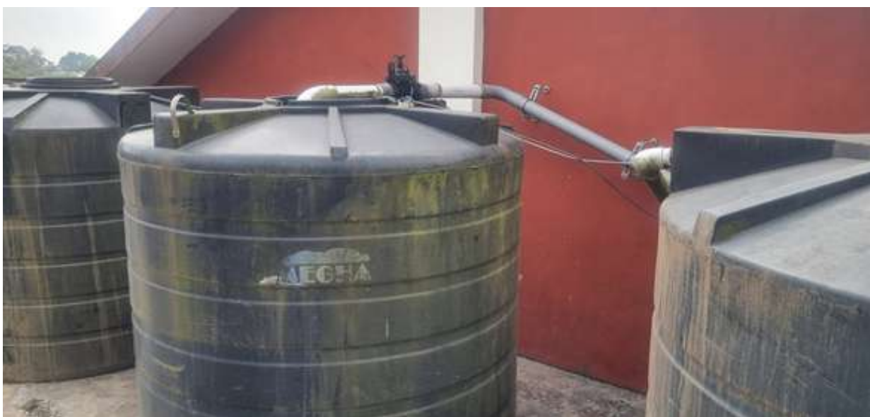
Fig 5.2 Water storage tank installed on campus
