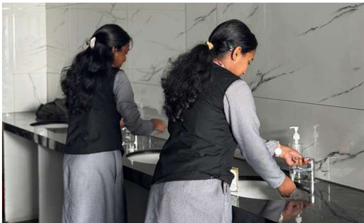
Fig 5.3 Water fixture installed in campus building
