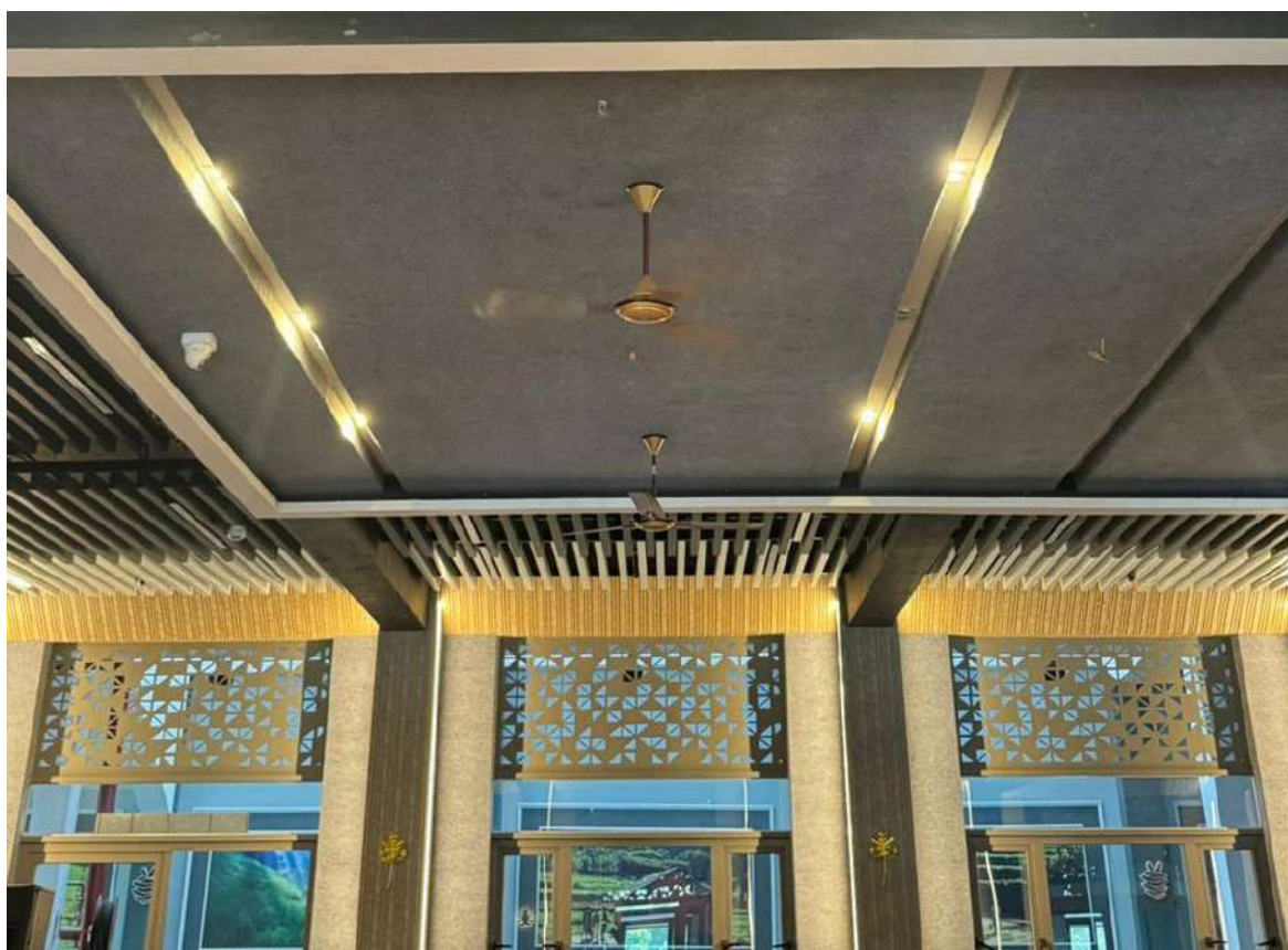
Fig 4.21 Electrical infrastructure of Auditorium -Magis Block
