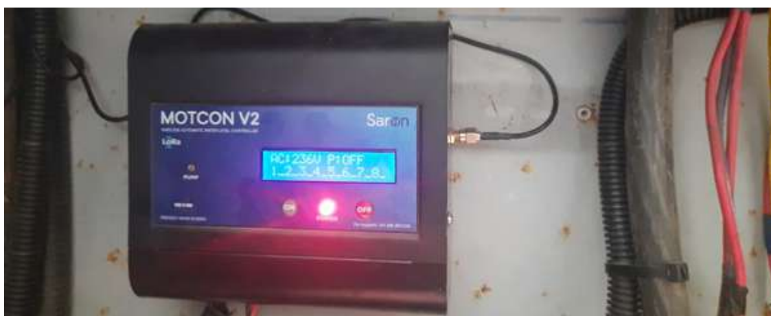
Fig 5.5 College water tank automatic filling and pumping mechanism
