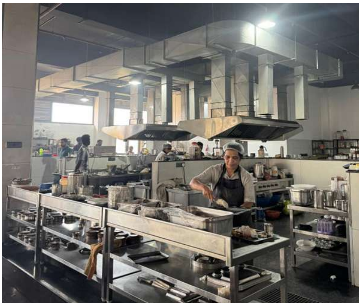
Fig 8.21 Main kitchen of the campus
