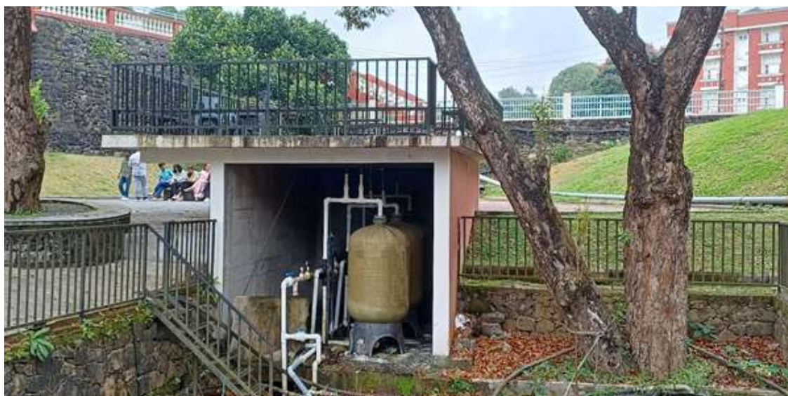
Fig 5.13 Water filtration unit of the campus
