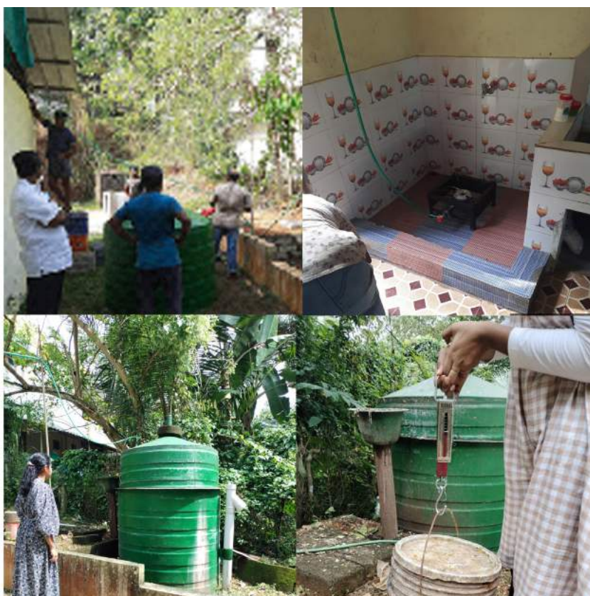
Installation of biogas plant at girls hostel and biogas is utilized for cooking purpose.
